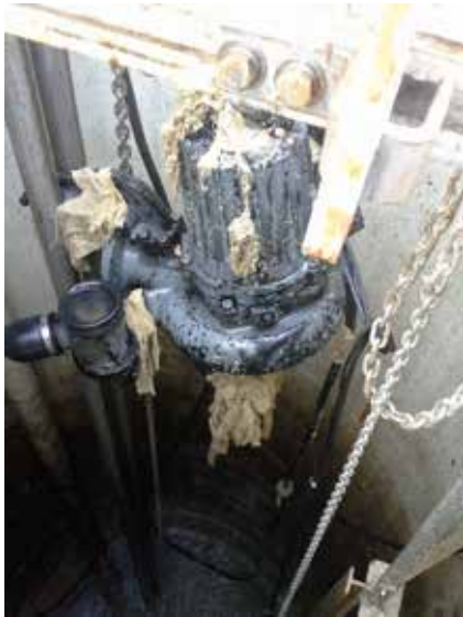
This picture came from the lift station at the corner of Sthitsem and Chowat rd, which receives septic materials from the following addresses:
