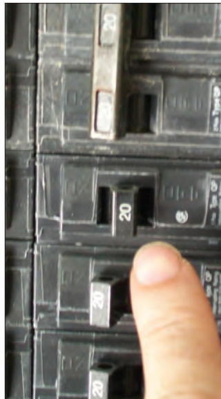
A tripped breaker will sit in the middle!
