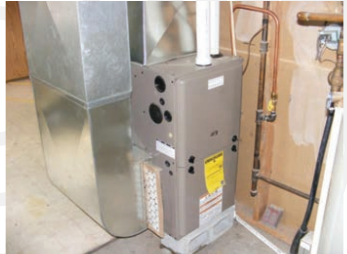
New appliances from retrofit completion
