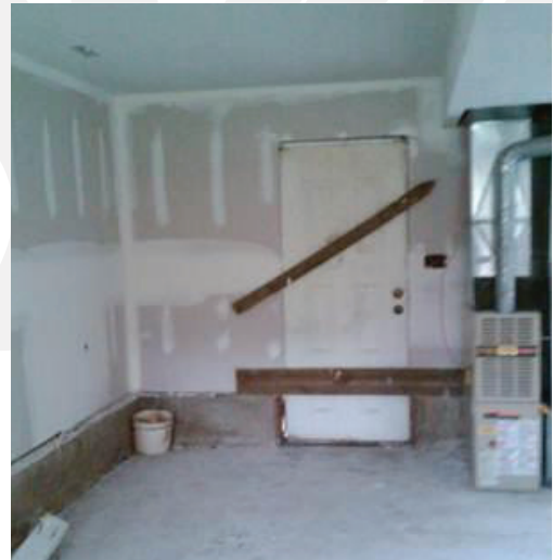
Damaged Unit Repair
