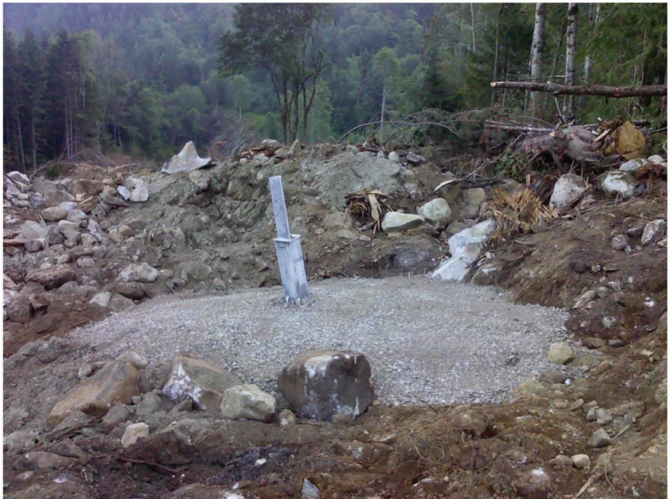
Figure 4: ILM Tower footing construction monitored by Seabird Island Heritage Monitor Conrad Louie.
