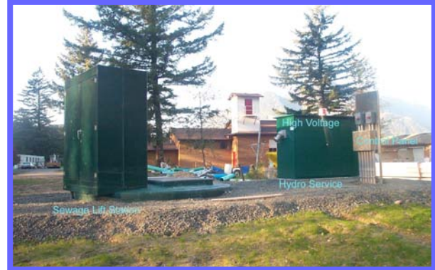
Lift station Behind Fire Hall
